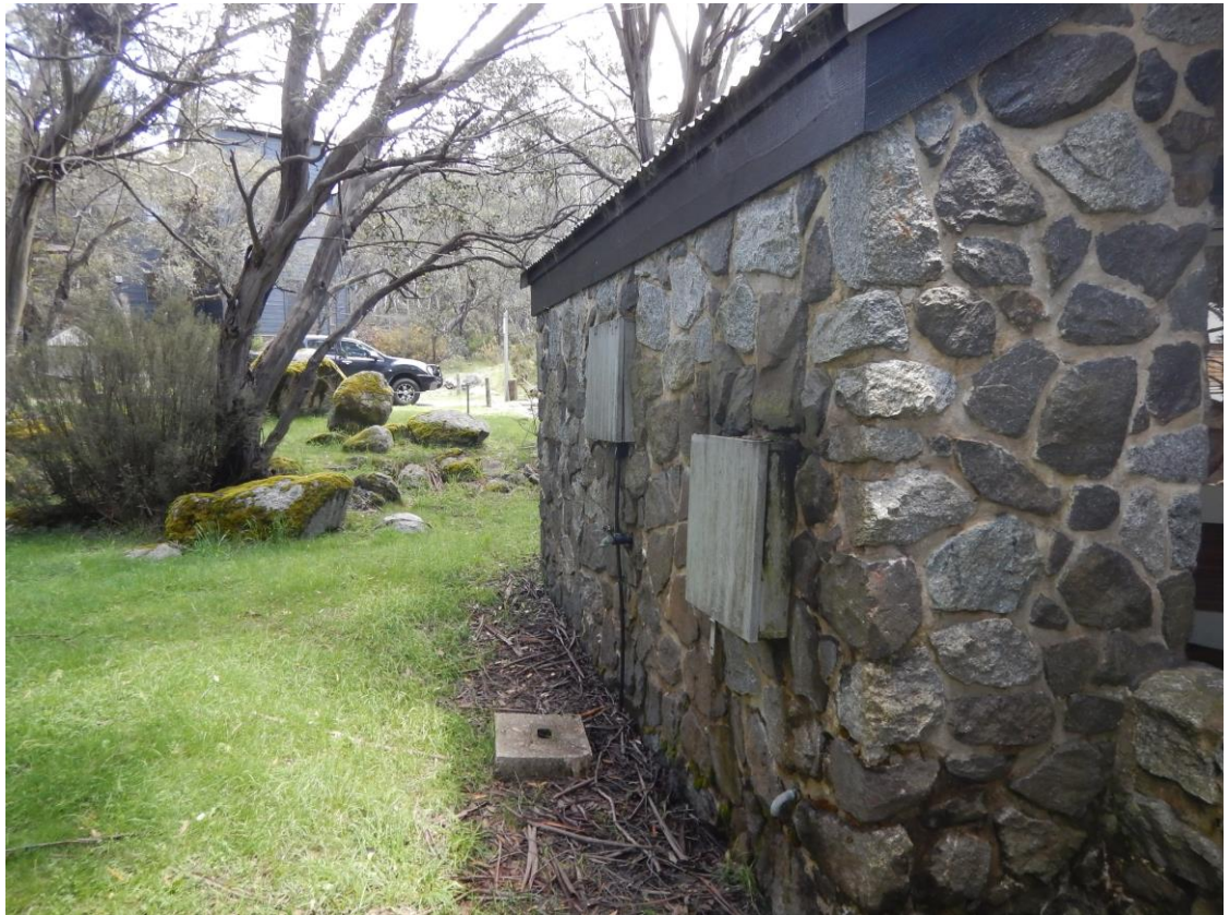
Figure 8: Photo showing the existing granite stone clad wall which will form the northern wall of the garage.
